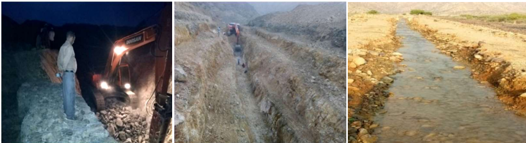
Figure 3: Partial view of main canal excavated by machine as well as human labor
